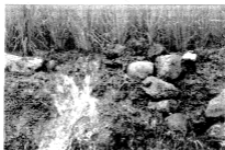
Figure 10: Eroded walls that cause irrigation waters to spill out (left of figure) are 'corked' using rocks (right of figure). (Photo taken July 31, 2009)
