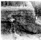
Figure 9: Leakage in terrace walls. (Photo Taken July 31, 2009)
